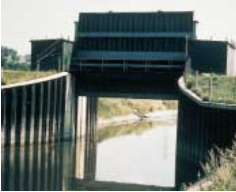
CANKLOW REGULATOR One of the control structures on the River Rother which helps to protect areas on the lower Don around Doncaster from flooding
