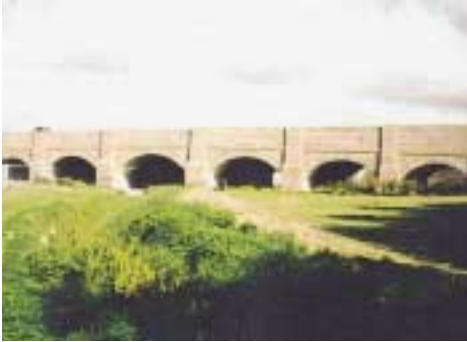
FLOOD ARCHES DONCASTER Flood water passing down the historical flood relief route flowed under these arches beneath the A638 Trunk Road.
