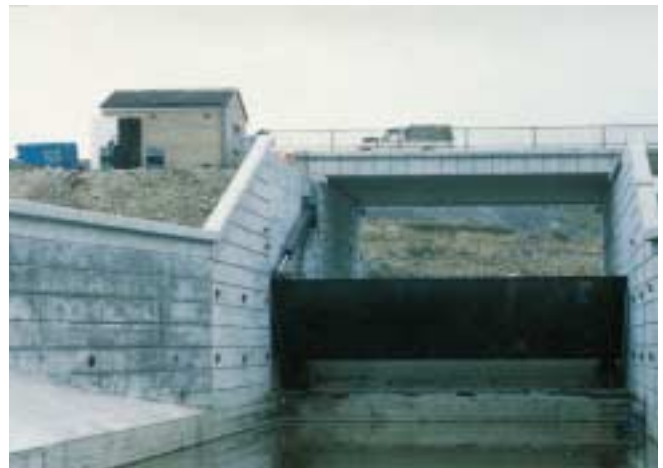
MEADOWGATE REGULATOR This regulator controls flood water on the Rother below Staveley and in extreme conditions helps to flood the washland areas which are part of the Rother Valley Country Park Complex
