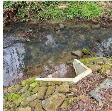
Treatment outlet - SE2998607525
